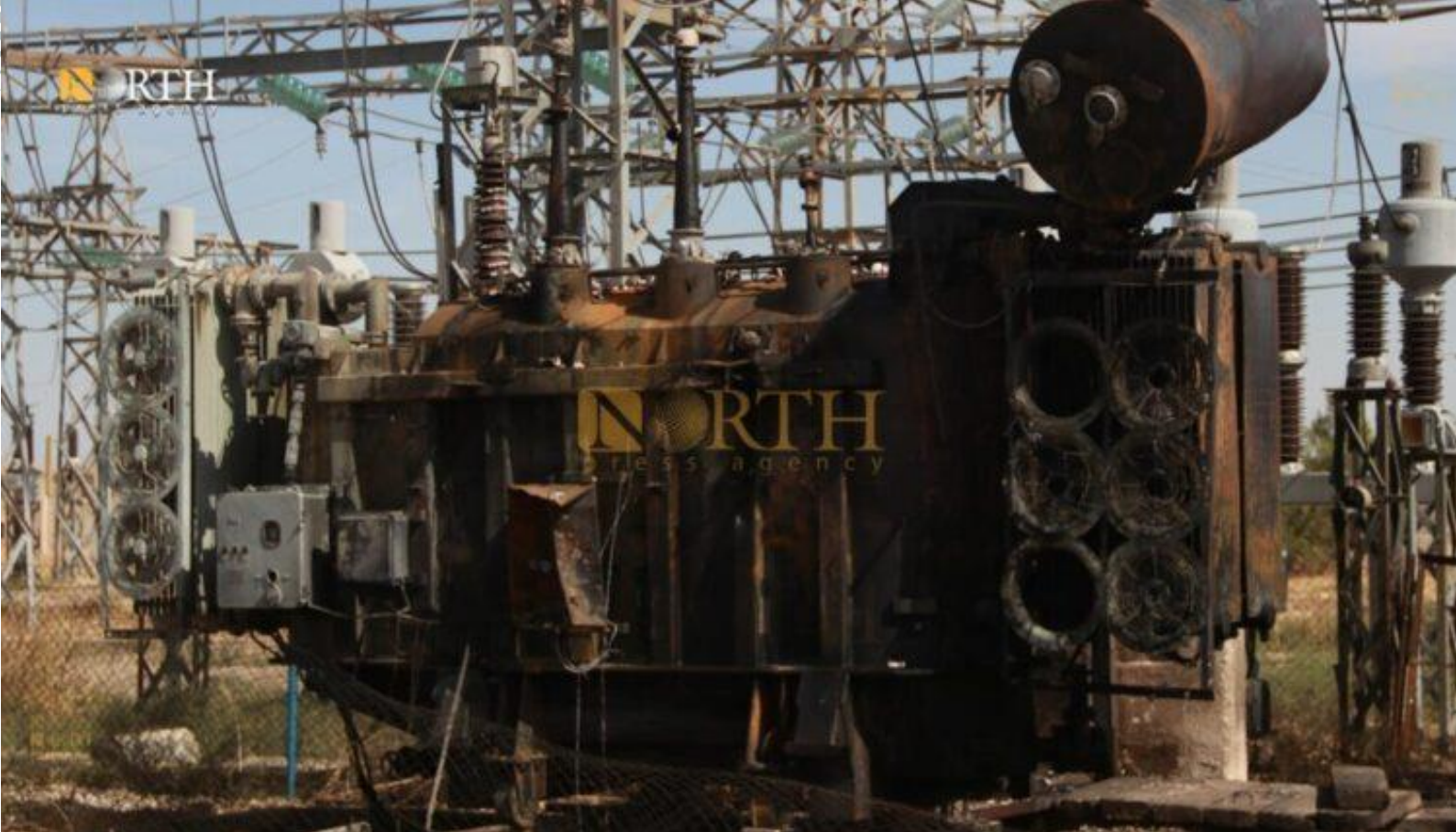
Image 2-Damage at the Amuda power transfer station caused by the Turkish airstrike on 5 October 2023. Source: North Press Agency .
