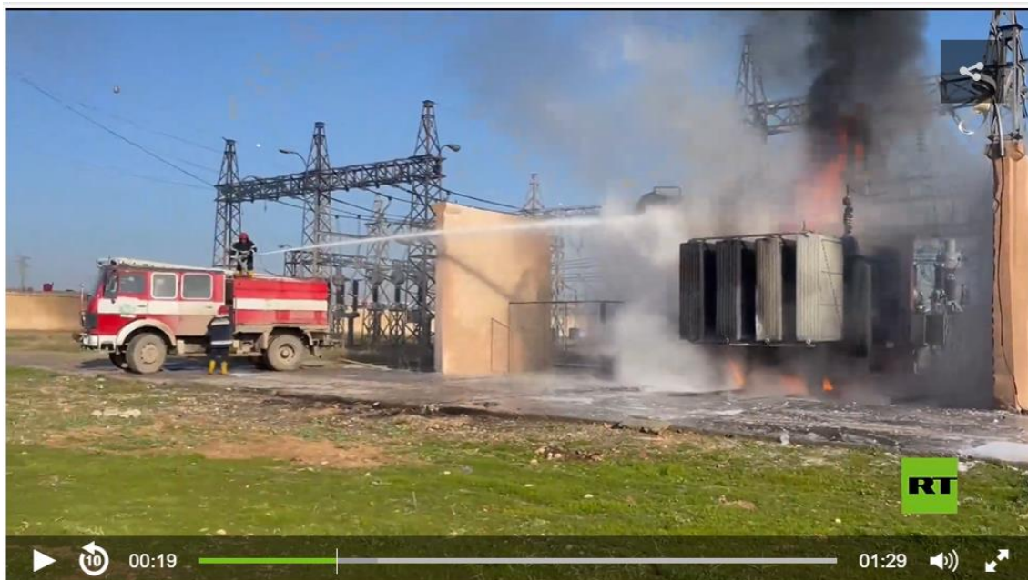
Image 16-Screenshot from a video documenting the condition of the power transfer station north of Qamishli/Qamishlo city following the Turkish airstrike on 14 January 2024. Source: Russia Today.
