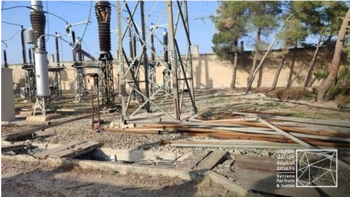
Image 7- A side of the damage caused to Sarmin power station by arterially shelling of 8 October 2023. Credit: The previous source.
