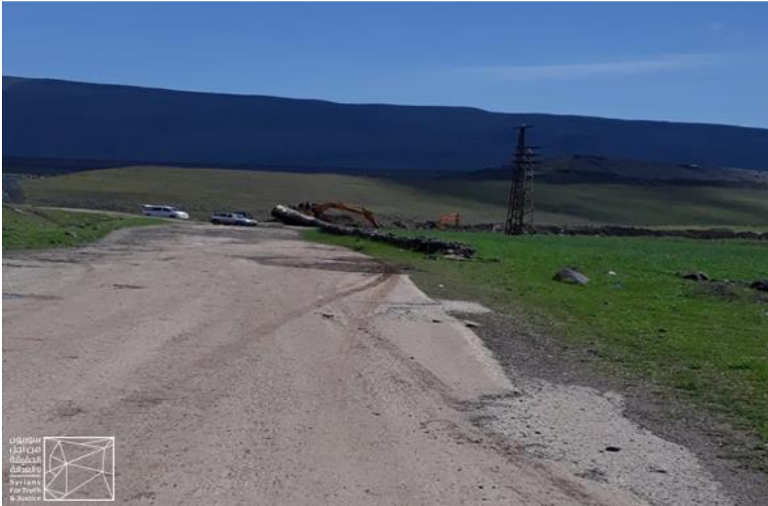
Image 3- a side of an area in the Ghab Plain dug by the TIP to remove water pipes. Credit: STJ.
