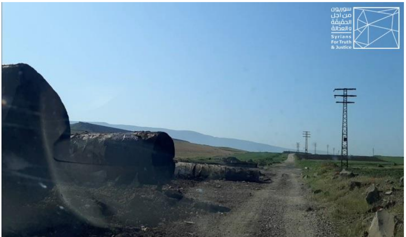
Image 6- a side of the removal of water pipes in the Ghab Plain. Credit: STJ.
