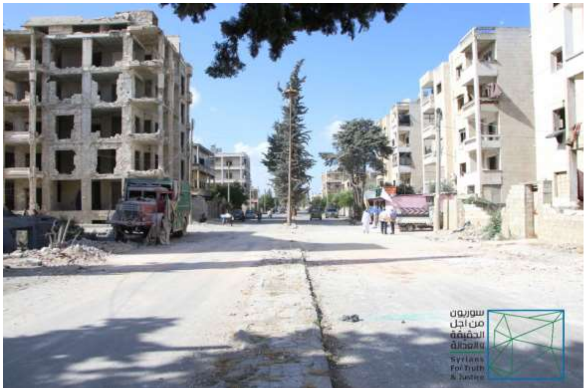
A residential building partially destroyed for being a target to air raids, Idlib city. Taken on: July 12, 2019. Photo credit: STJ.
