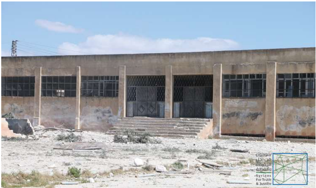
The damage caused to one of Kansafra schools on June 4, 2019. Photo credit: STJ.
