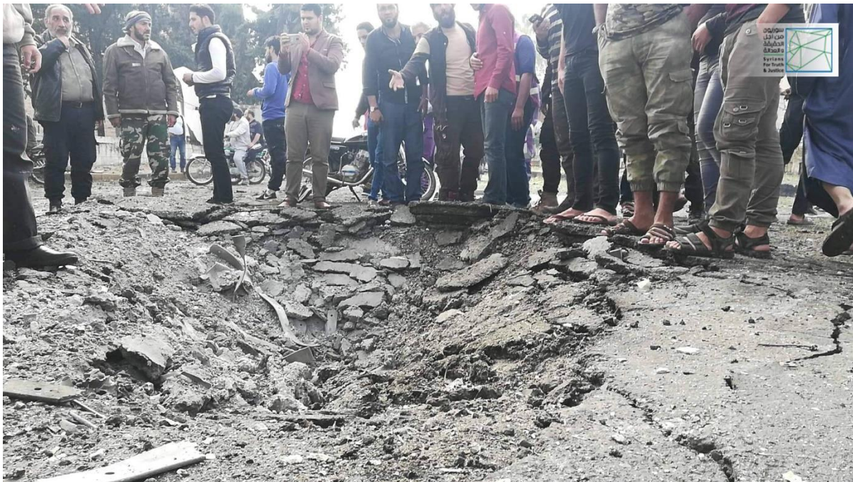
A hole in the street caused by a car bomb explosion in the al-Qusour neighborhood, Idlib city. Taken on: October 21, 2018. Photo credit: STJ.
