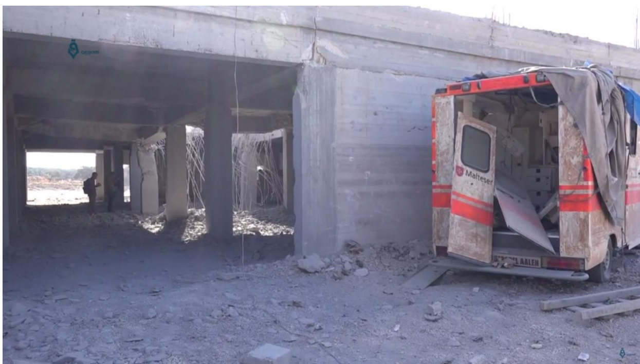
Photo showing the damage in one of the ambulances and it shows the big hole formed from the missile in the back – Source: Video for “Qasyun” news
