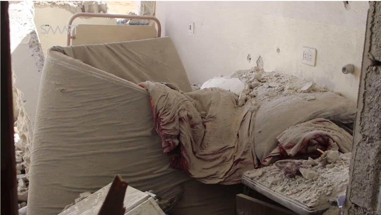
Photo showing the damage in the hospital – Source: Video for “Smart” media agency
