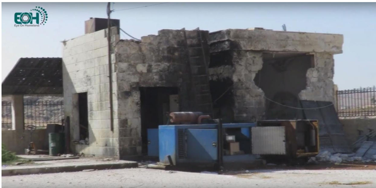
Picture showing the destruction of the generators in the northern western side of the hospital – Source: Video of “Ain ala alwatan” media agency
