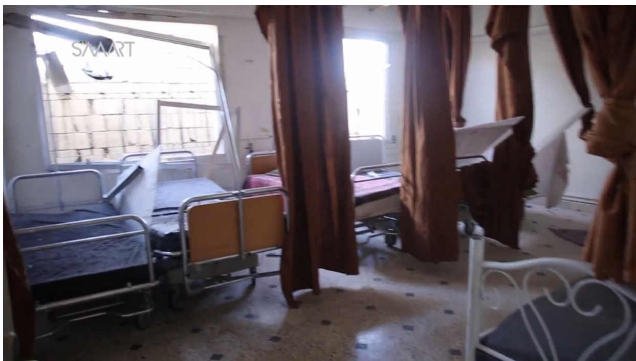
Picture showing some physical damage in the hospital – Source: Video for “Smart” media agency
