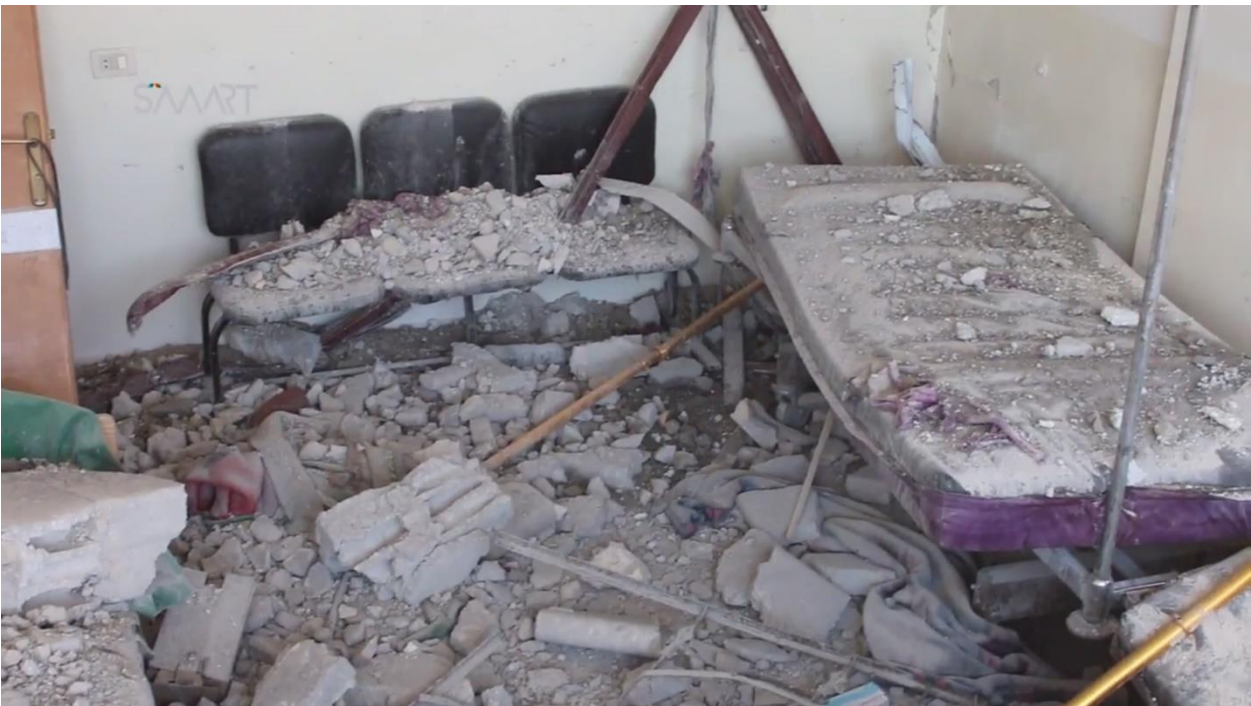
Photo showing the damage in the hospital – Source: Video for “Smart” media agency
