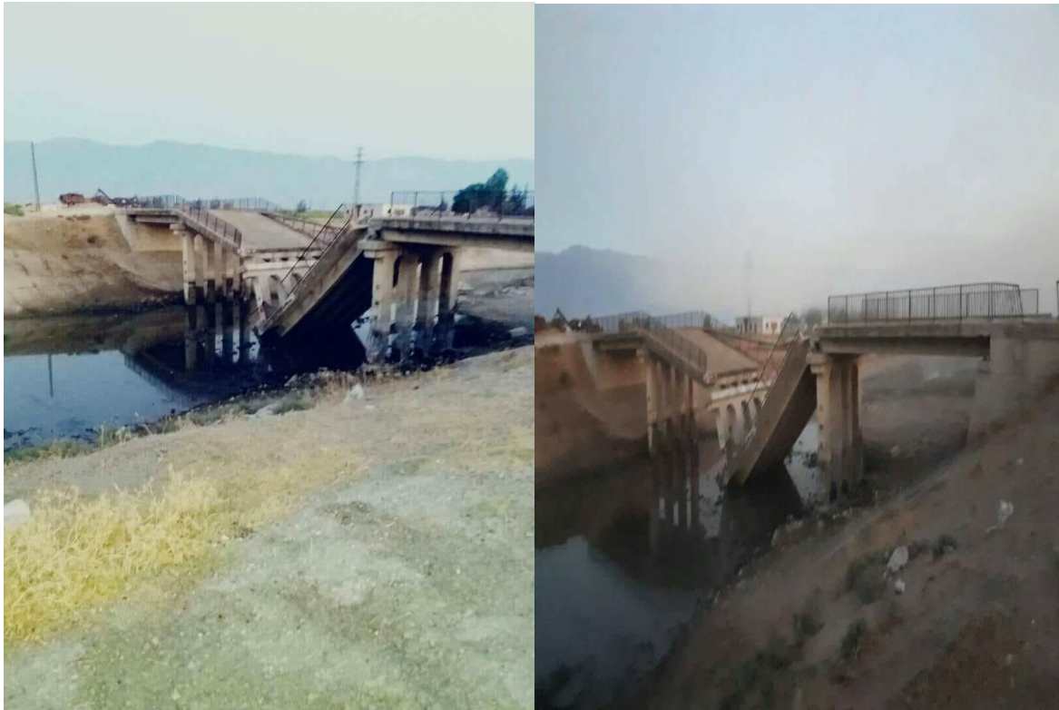
Bait al-Ras and al-Sharia bridges in Sahl al-Ghab after being bombed by the National Front for Liberation on August 31, 2018.
