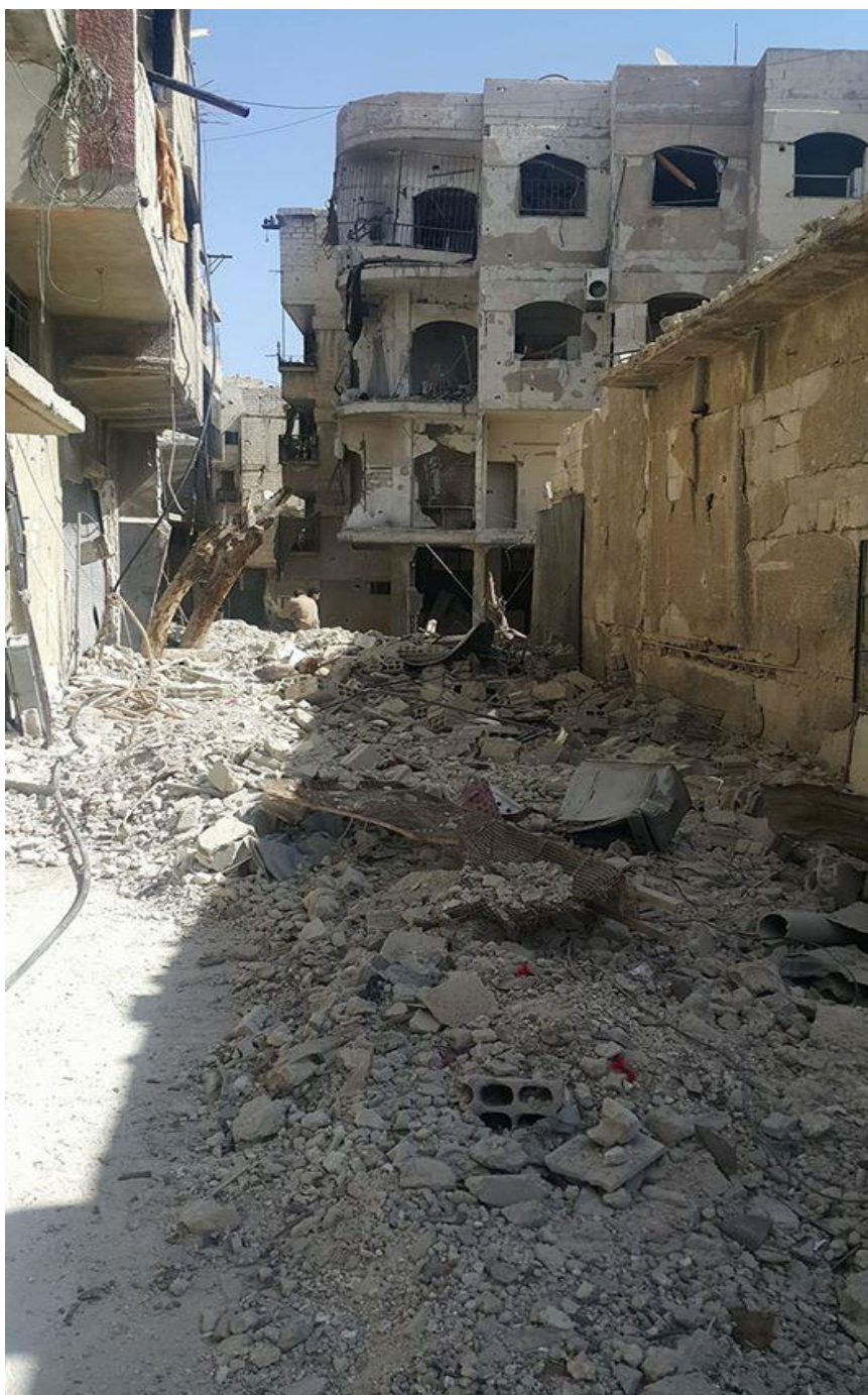
An image shows an aspect of the destruction of the house of Iyad al-Ali, the witness, following an aerial bombardment on February 21, 2018.
