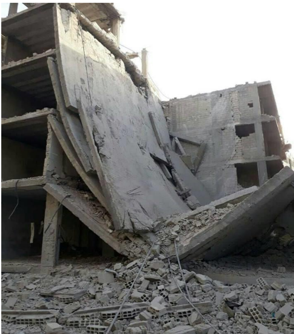
An image shows part of the destruction of civilians' homes in Hamoryah City, following the bombardment in March 2018.
