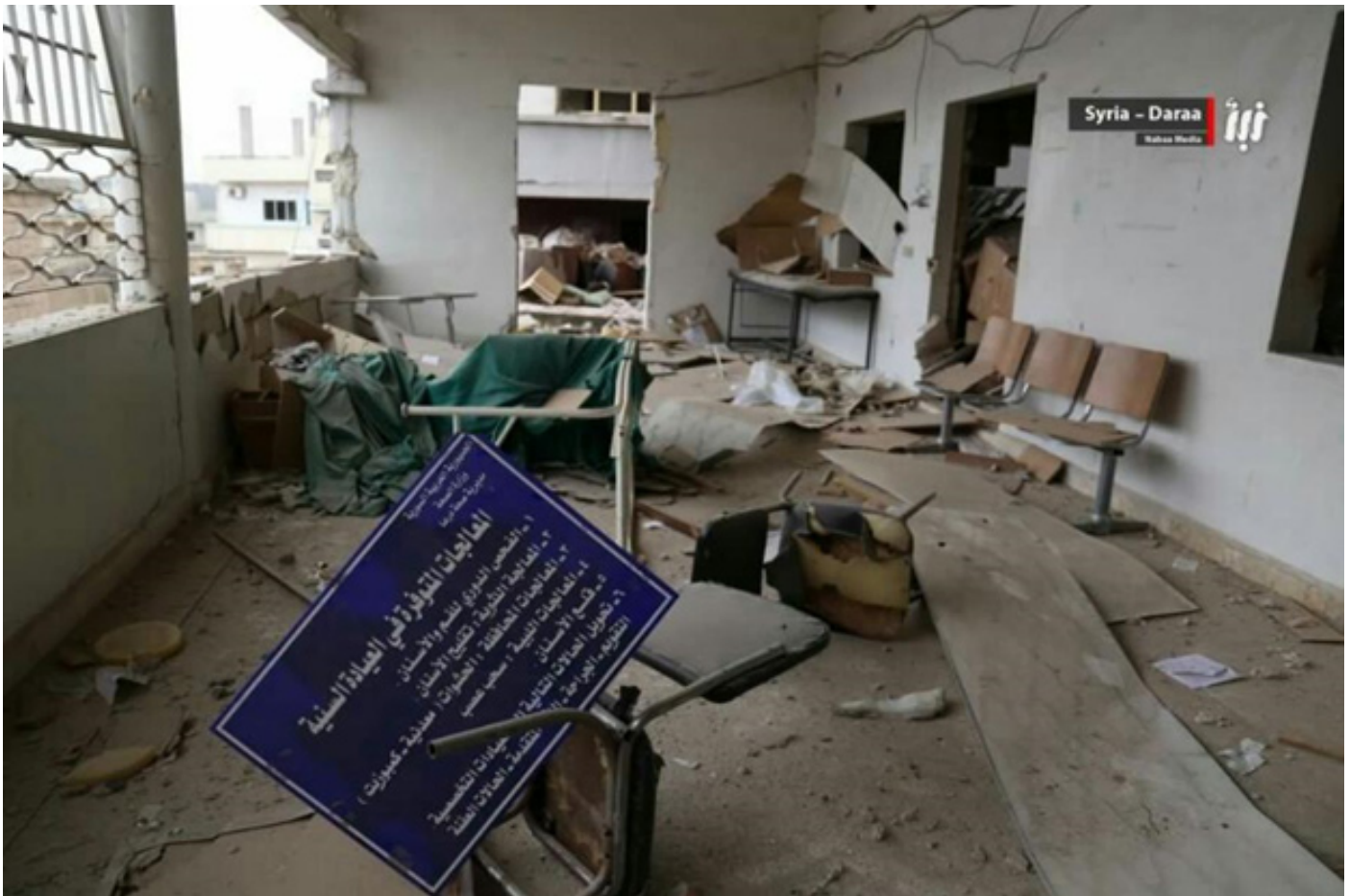
.Image showing the damage to Daraa al-Balad hospital due to the airstrikes Photo credit: Nabaa Media Foundation
