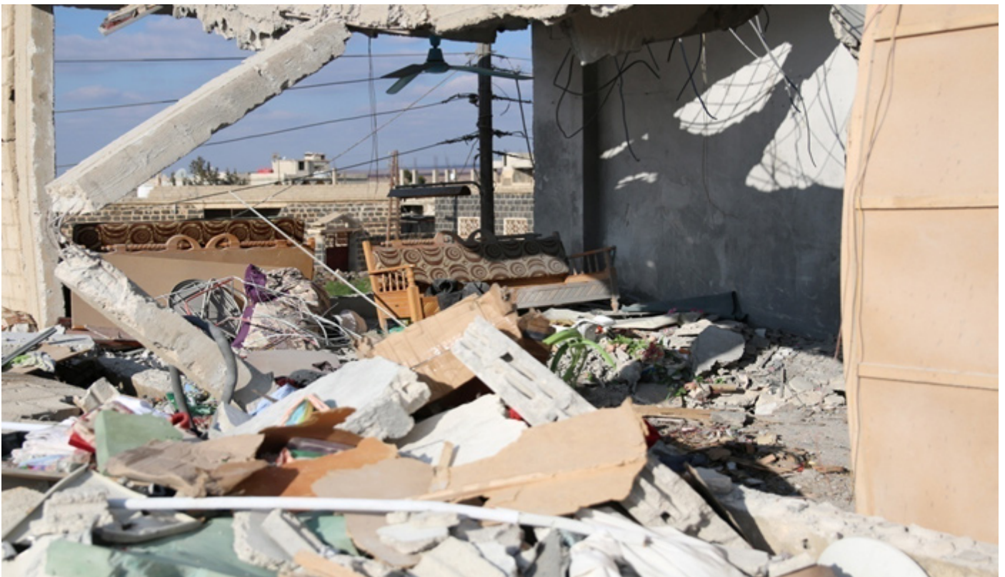
Image showing destruction caused to civilian houses in the Russian airstrikes on Busra al-sham Photo credit: Alaa al-Faqir
