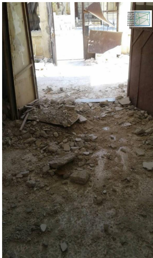
The destruction caused to the witness Mohammed Abdulaziz Othman's house following shelling Zayzoun town, Hama countryside on August 12, 2018.
