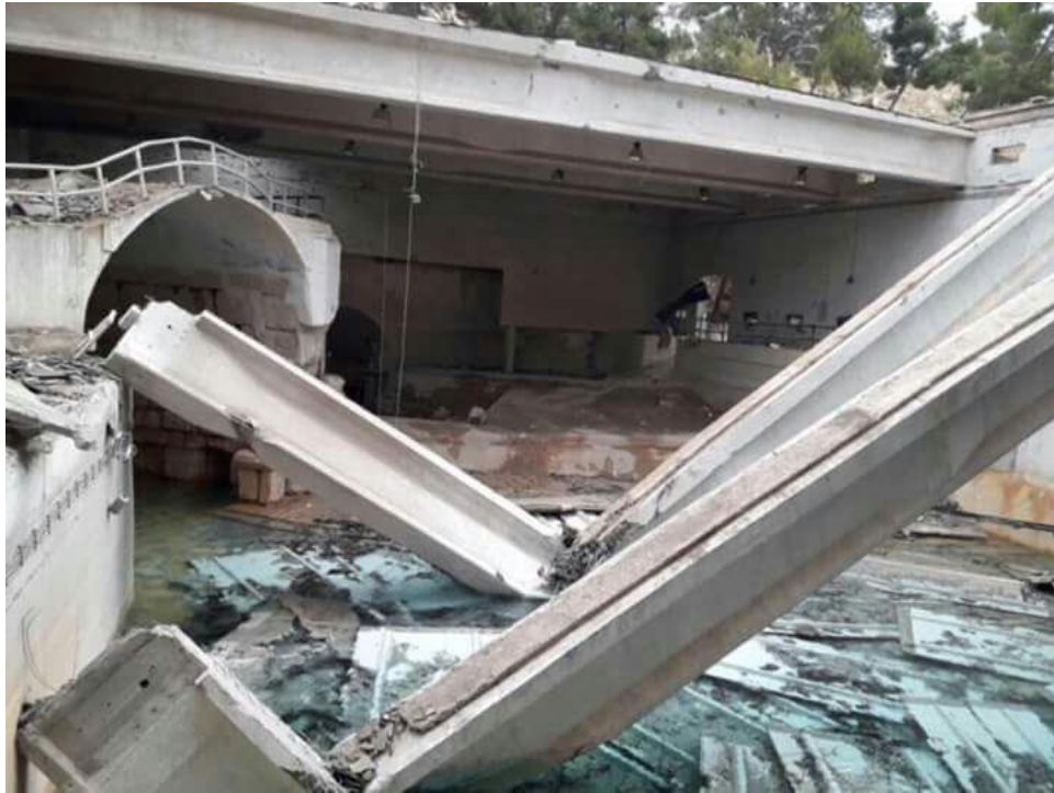
Images illustrating the damage caused to Ein-al-Fejeh facility as a result of bombing by regime forces.
