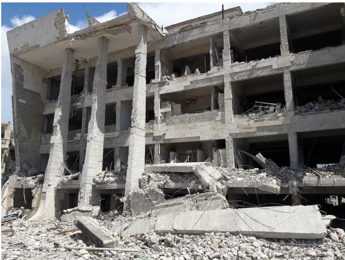
An image shows some of the devastation in the middle of Idlib city following the explosion on May 12, 2018. Photo credit: STJ
