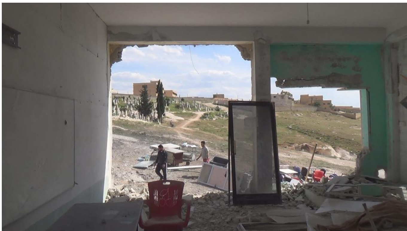
An image shows an aspect of the destruction of the medical center in Kafr Sijnah, following shelling it with barrel bombs on April 25, 2018. Photo credit: STJ
